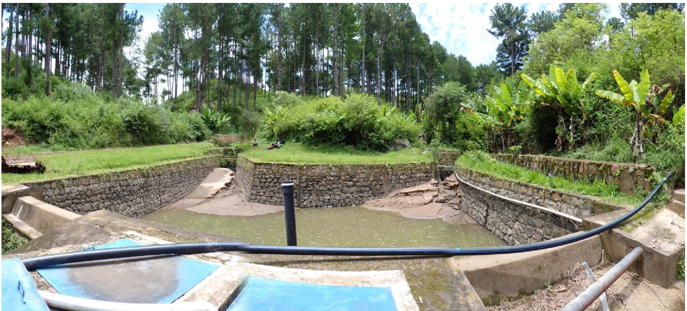
Figure 11. Diversion dam feeding Analavory city, showing extensive sediment buildup
